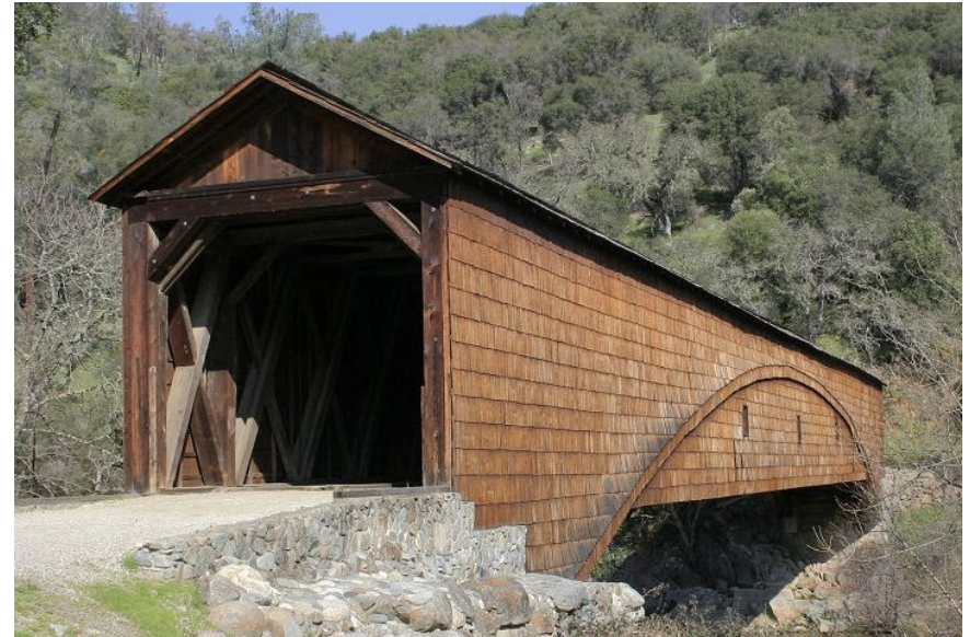
In the 1850s and 60s, thousands of loaded wagons crossed the South Yuba River at Bridgeport en route to California and Nevada mines. The 1862 bridge is the longest single-span covered bridge in the United States.
